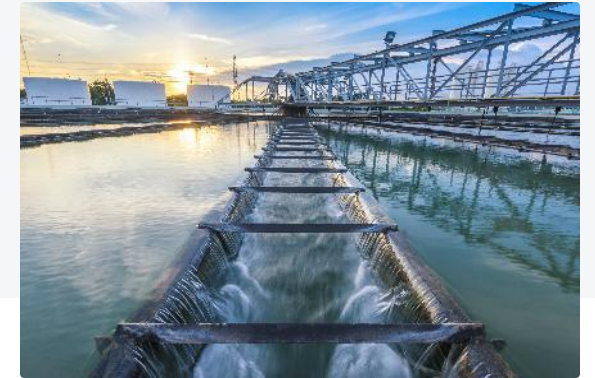
Low disinfection residual
