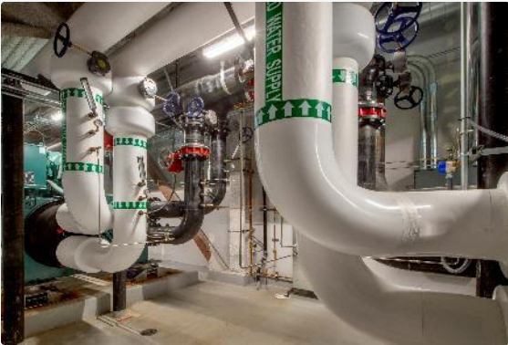
Complex plumbing systems
